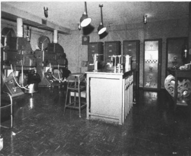
Magnetic reproducing equipment in the motion picture theater. Ampex installation along the far wall (at Warner Theater, New York City) provides six channel stereophonic sound.
